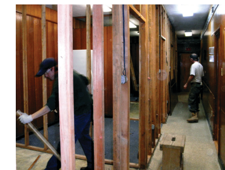
And the walls come down carefully through the skill of Andrew and Ed. Note the confinement of the long-time pantry area and the congestion that staff and volunteers needed to negotiate while filling menus.
