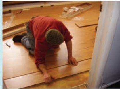
Robert installs new flooring in Marylou's office with the help of Richard and Brian
